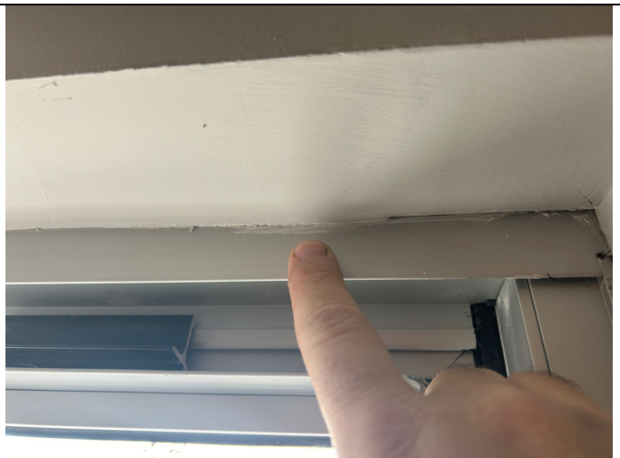
Paint on window frame in Unit 212. This is a typical condition.
