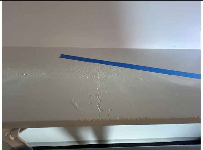
Visible side of wood shelf in bedroom closet at Unit 214.
