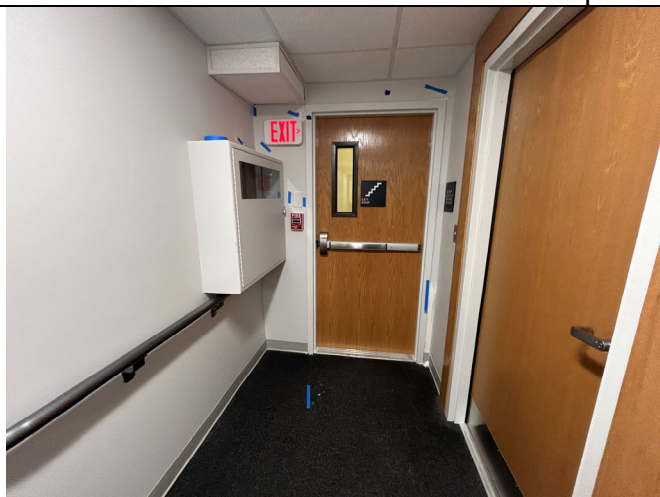
South stairwell door with gypsum board finish deficiencies identified w/ blue tape.
