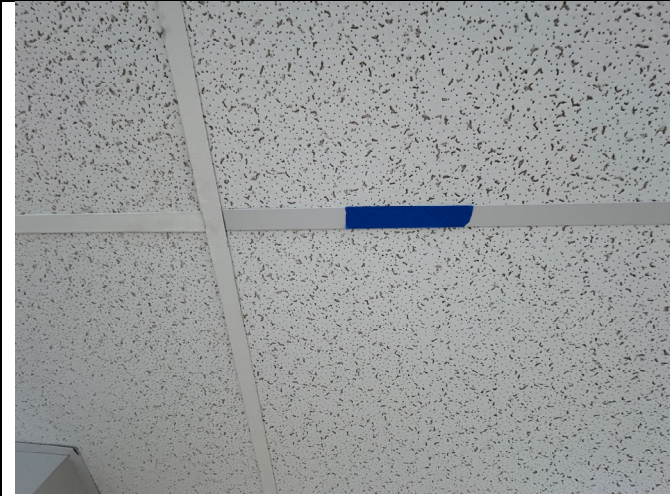
Infill T-grid not the same color as painted grid in Common Space 208.
