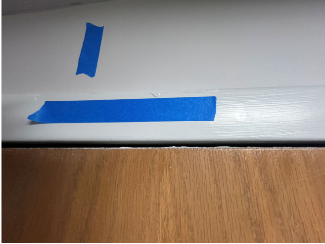
Paint drip & heavy brush strokes visible above jan closet door in corridor.
