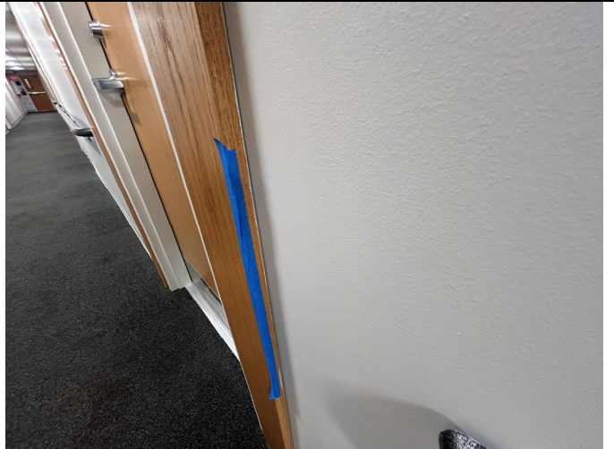
Paint to be removed from wood trim at a typical unit entry door in corridor.
