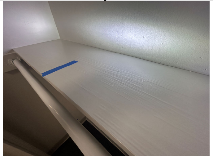
Wood shelf installed upside down in closet of Unit 209. Typical in multiple units.
