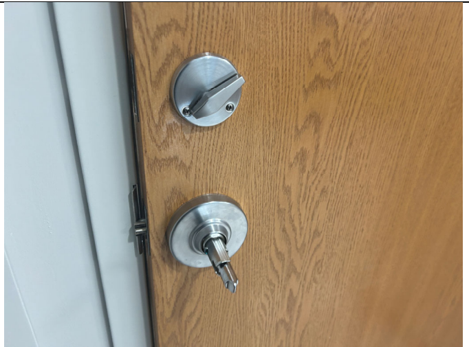
Lockset door handle in Unit 214 to be secured.
