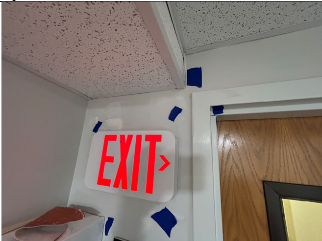
Gypsum board finish touch-up and paint required in north corridor above stairwell door.
