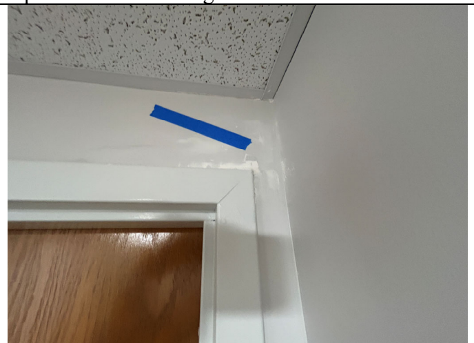
Gypsum board finish touch-up and paint required in south corridor above stairwell door.
