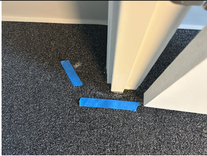
Paint on carpet in Bedroom 2 closet in Unit 211.
