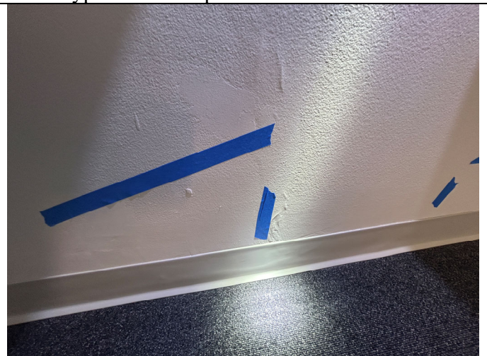
Condition at existing wall in Unit 207 that has not been finished to "like new" condition.
