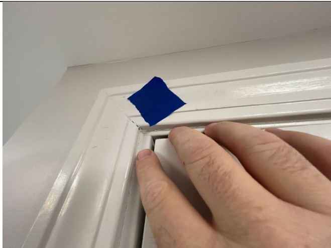
Wood door frame requiring additional wood filler, sanding, and repainting. Typical in various units.
