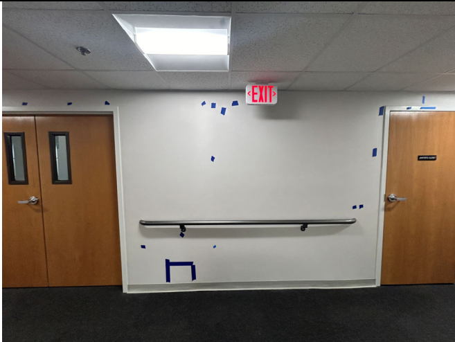
Gypsum board finish deficiencies identified w/ blue tape in corridor between Doors A-207 & A-208.
