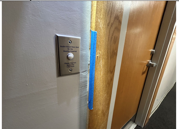
Gypsum board finish touch-up and paint required adjacent to unity entry door at Unit 201.
