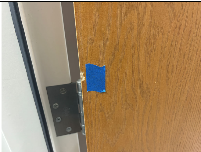
Damaged wood veneer to unit entry door at Unit 214.
