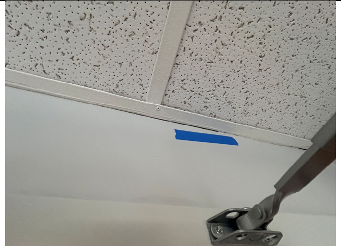
Gap at existing ceiling wall angle requiring caulking & paint in Common Space 208.
