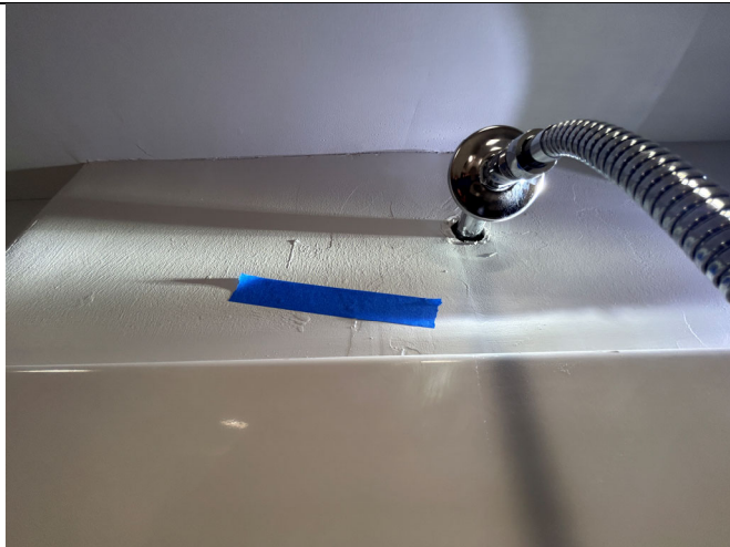
Deficient gypsum board finish at shower head in Unit 214.
