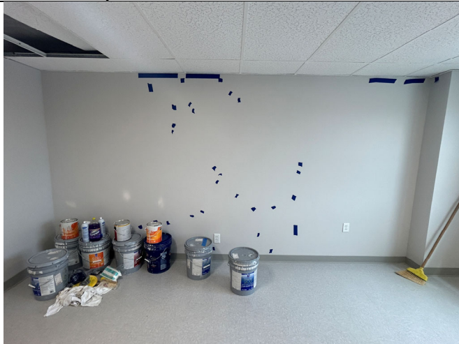
North wall of Common Space 208 with gypsum board finish deficiencies identified w/ blue tape.
